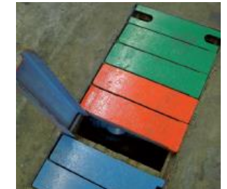
Technical duct on the floor
