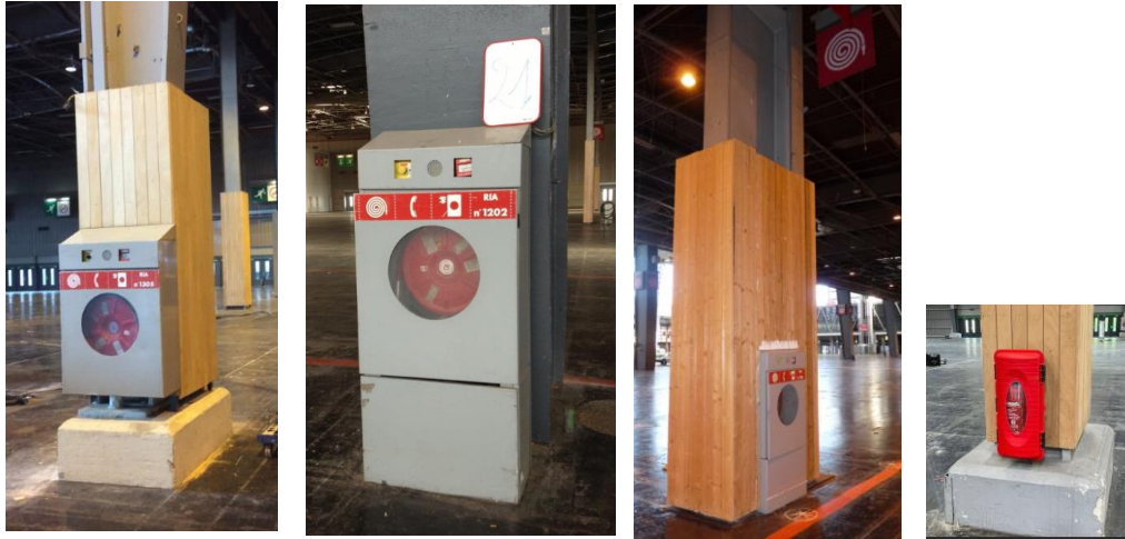
FIRE HOSE REELS
