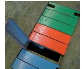
Technical duct on the floor
