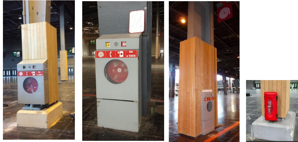
FIRE HOSE REELS
